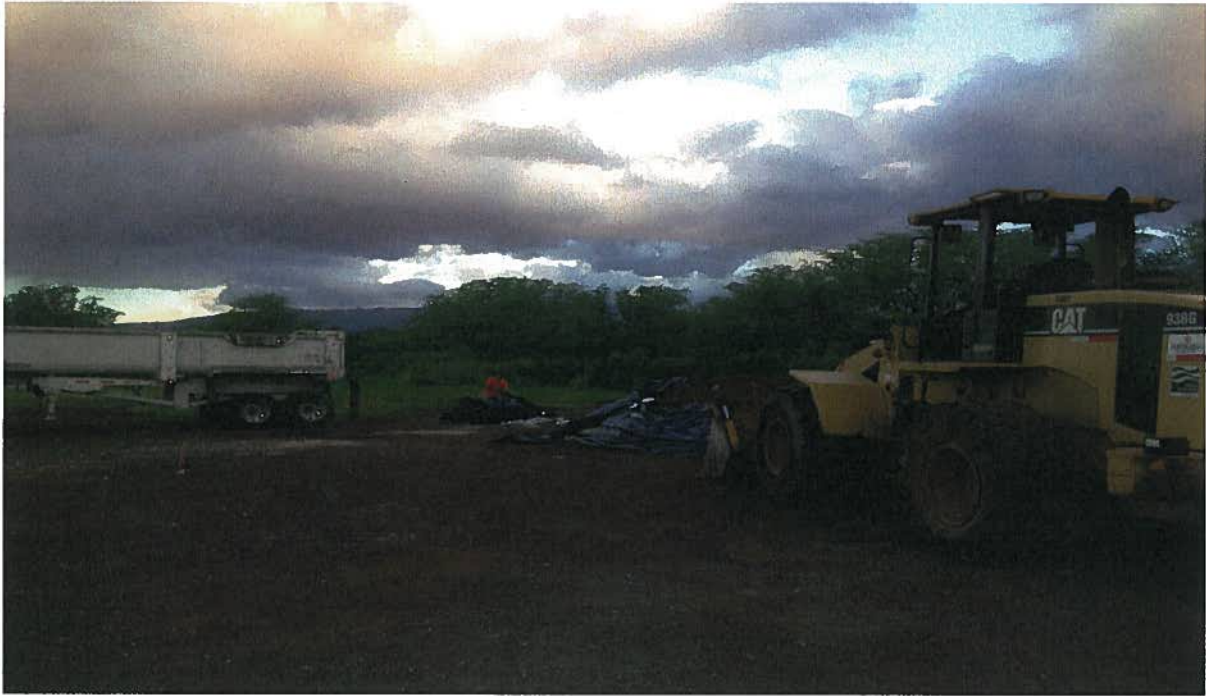
Photo 11. Removed Plastic Cover from Contaminated Soil Stockpile
